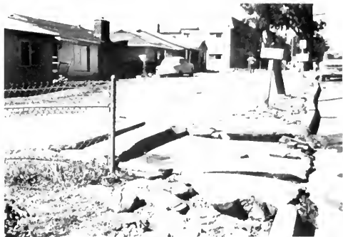
Photo 16. Surface break of Sylmar segment of San Fernando fault zone extends northwest along edge of Foothill Boulevard toward houses and modern apartment building (photo 15). In foreground, concrete driveway and its asphalt approach to boulevard were broken into short segments which were successively overthrust. In February 1972, house next to site of apartment was jacked-up, and a new foundation was constructed beneath it; severely damaged middle house was unoccupied.
